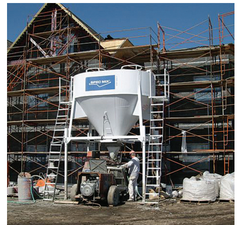
SPEC MIX silo system improves production and mix consistency and eliminates the disposal of wasted sand and bagged goods
